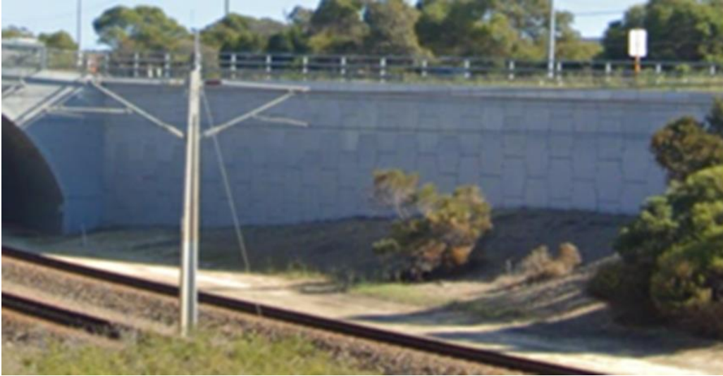
Figure 8 Steel Barrier on Top of the Retaining Wall Protecting the Rail Corridor from Vehicles Travelling on the Freeway
