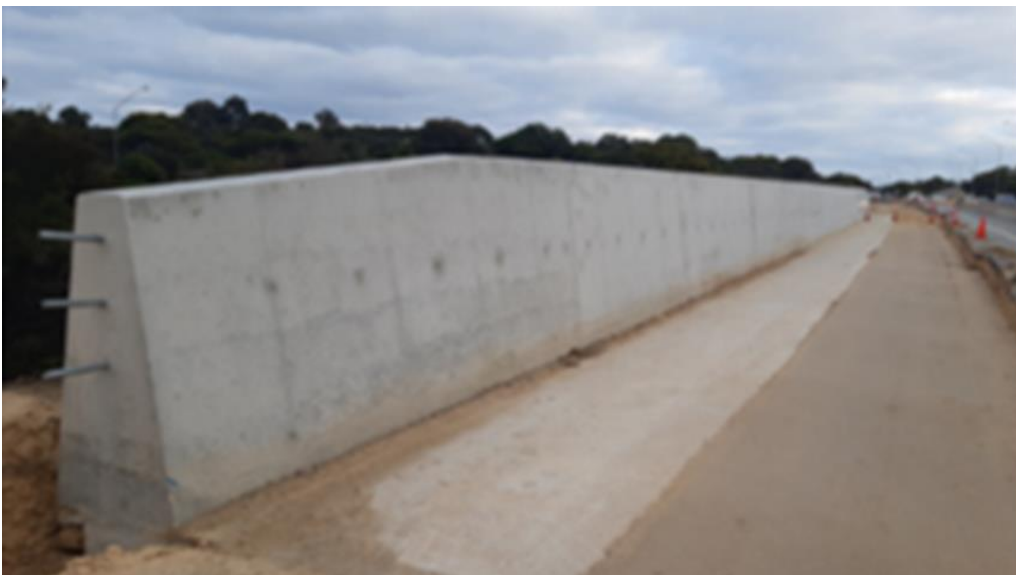
Figure 9 The Steel Barrier on Top of the Retaining Wall has been Removed and Replaced with the Concrete Structure Seen in the Image Above
