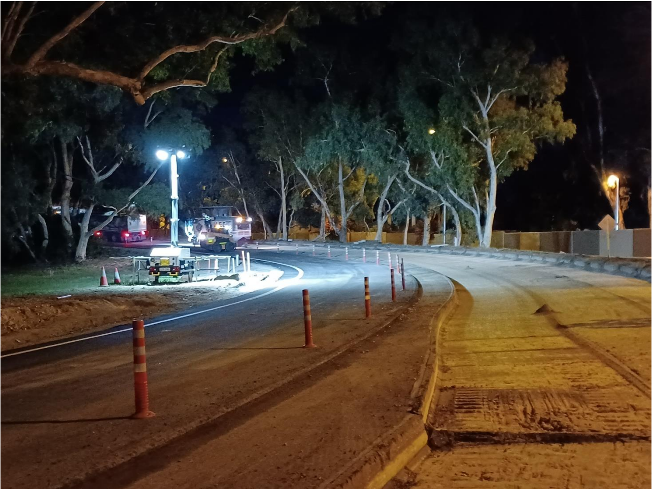
Figure 9 Solar Lighting Tower in Use
